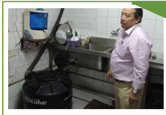
Owner with waterwaste collection tank at underground kitchen at a hotel.
