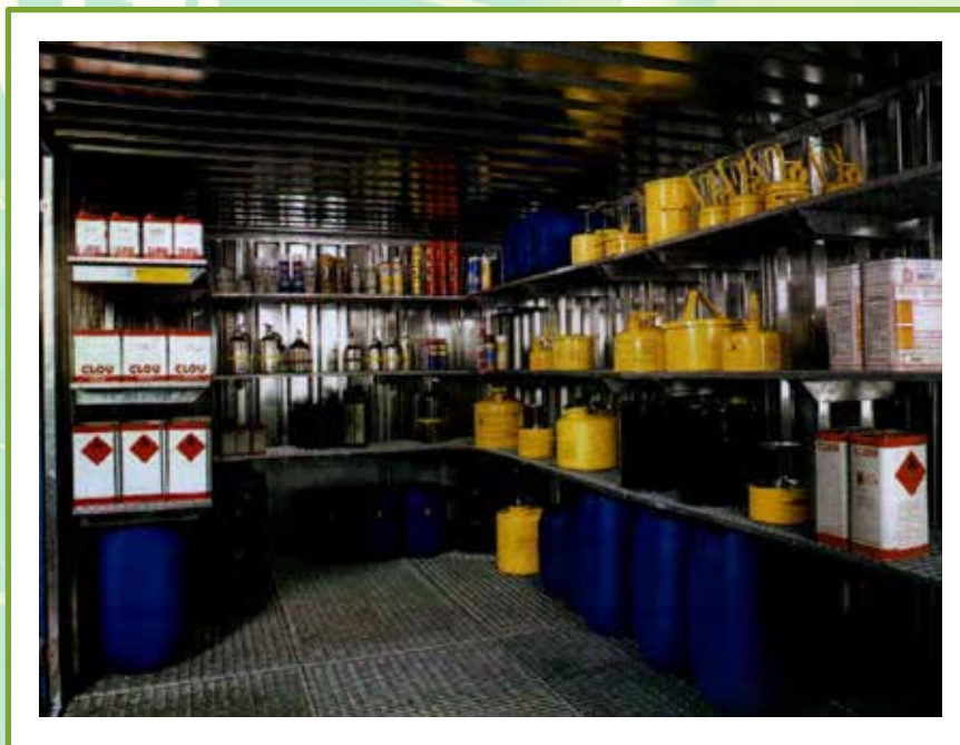
Proper chemical storage with strong shelves, proper separation, and drip tray
