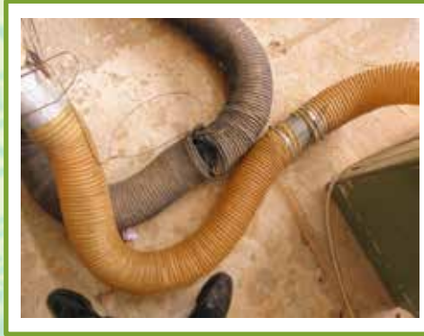
Duct to transfer dust to a silo
