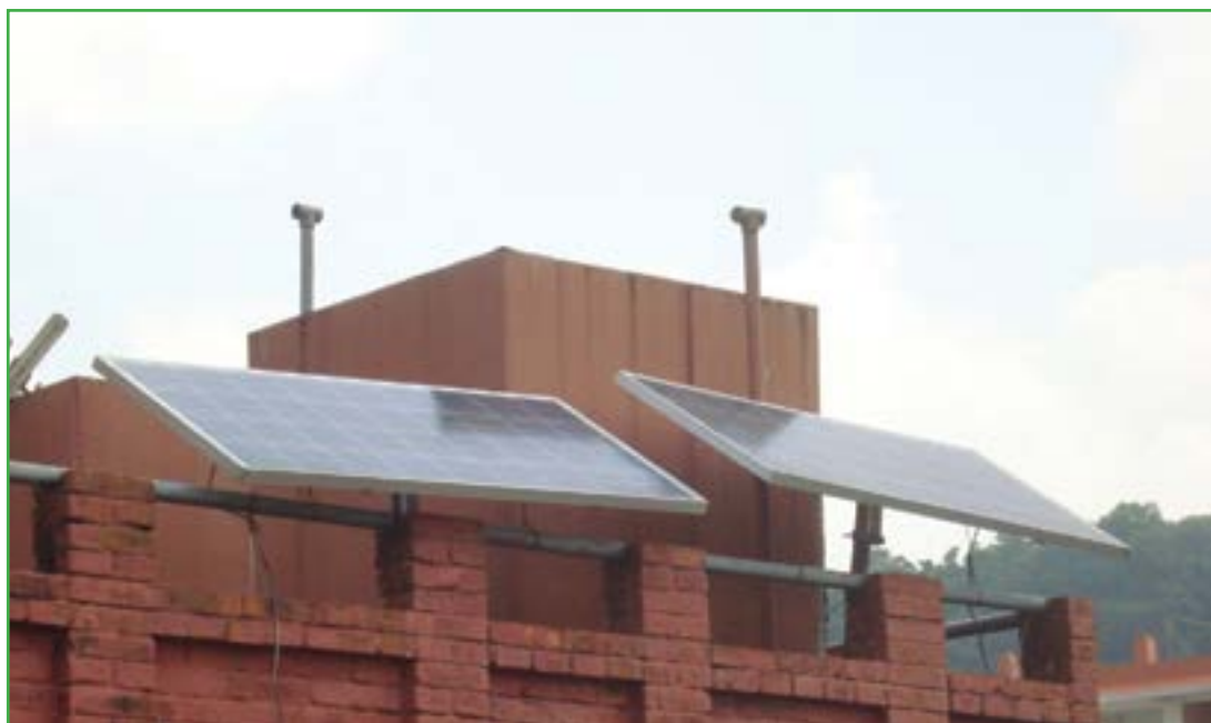
Solar PV (2 x 140 watt) installed at Fairmount Hotel, Pokhara
