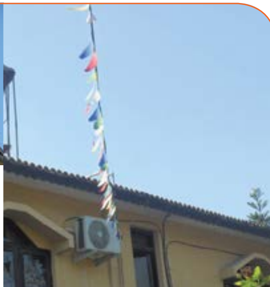
AC compressor placed on rooftop and exposed to direct sunlight (on left) & AC compressor placed on the north wall, avoiding direct sunlight (on right)
