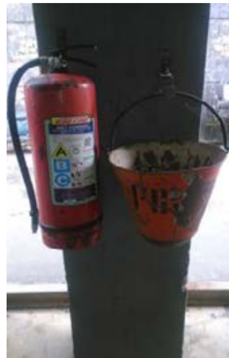
Fire extinguisher in place
