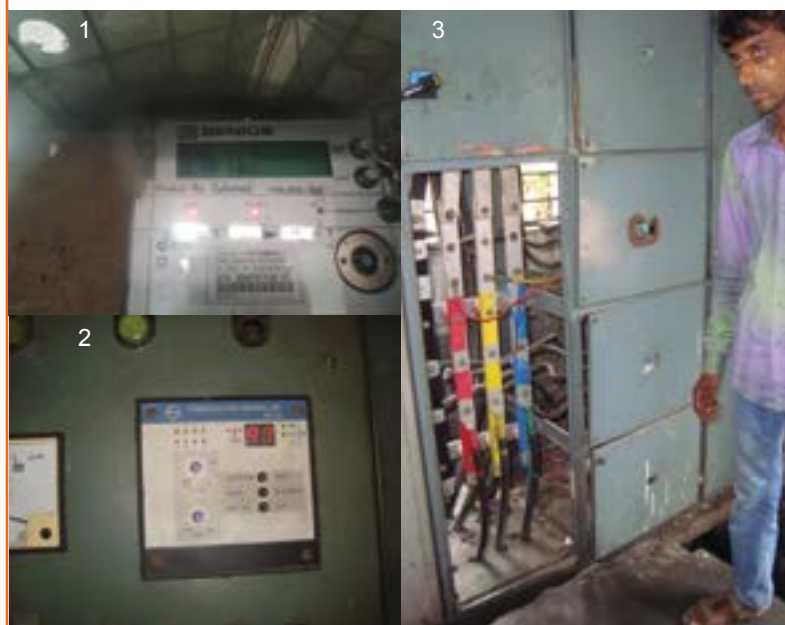
1 Power factor during initial assessment. 2 Corrected power factor. 3 After maintenance of electrical connections
