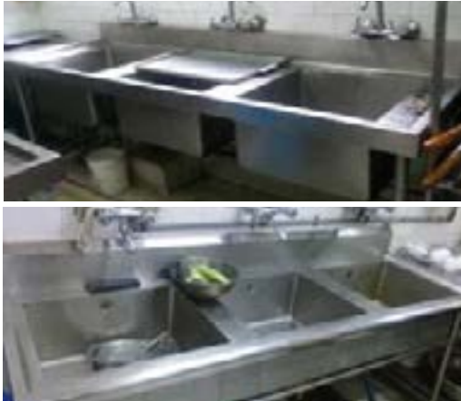
The hotel staff started making effective use of the sink system which was already in place
