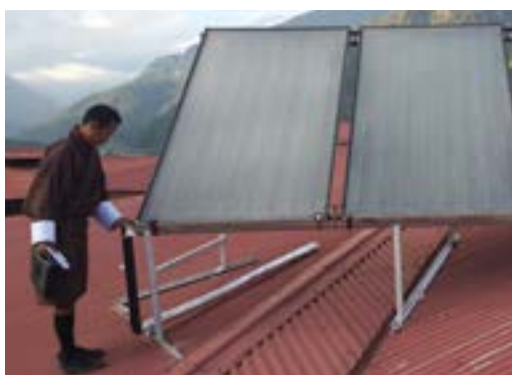
Solar panels installed on the roof
