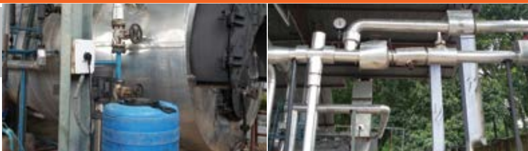
Insulation of boiler surface and steam pipelines
