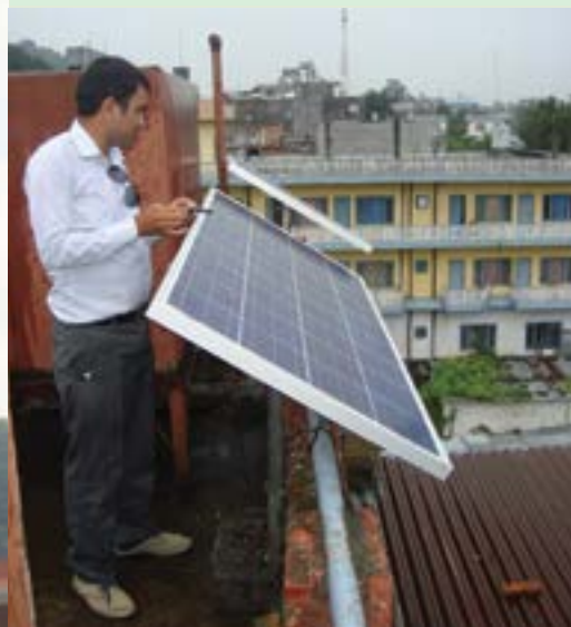
SEID local consultant checking the orientation of solar PV at Fairmount Hotel, Pokhara
