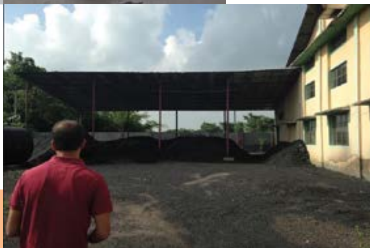
Construction of an awning to protect coal from rain (above: before; below: after)
