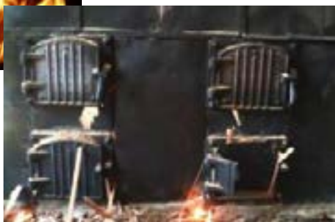
The furnace doors are closed during combustion
