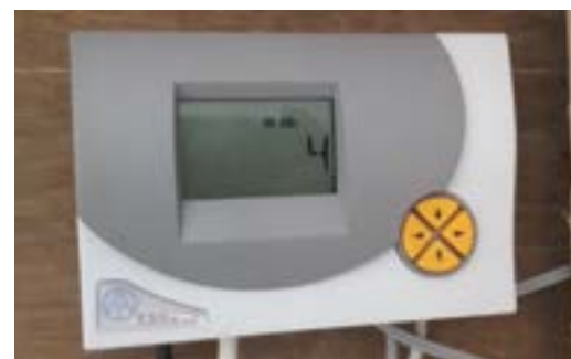
Control panel showing thermal power generated by the solar water heater
